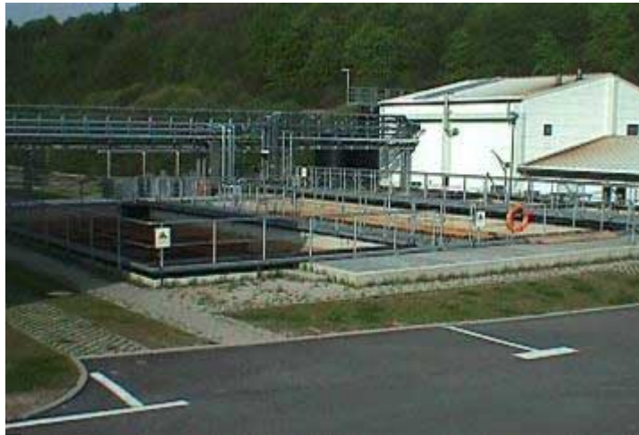
Mine water treatment facility of WISMUT at Schlema-Alberoda
